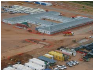
Mei Hitachi, Medupi Power Station 3000m 2
